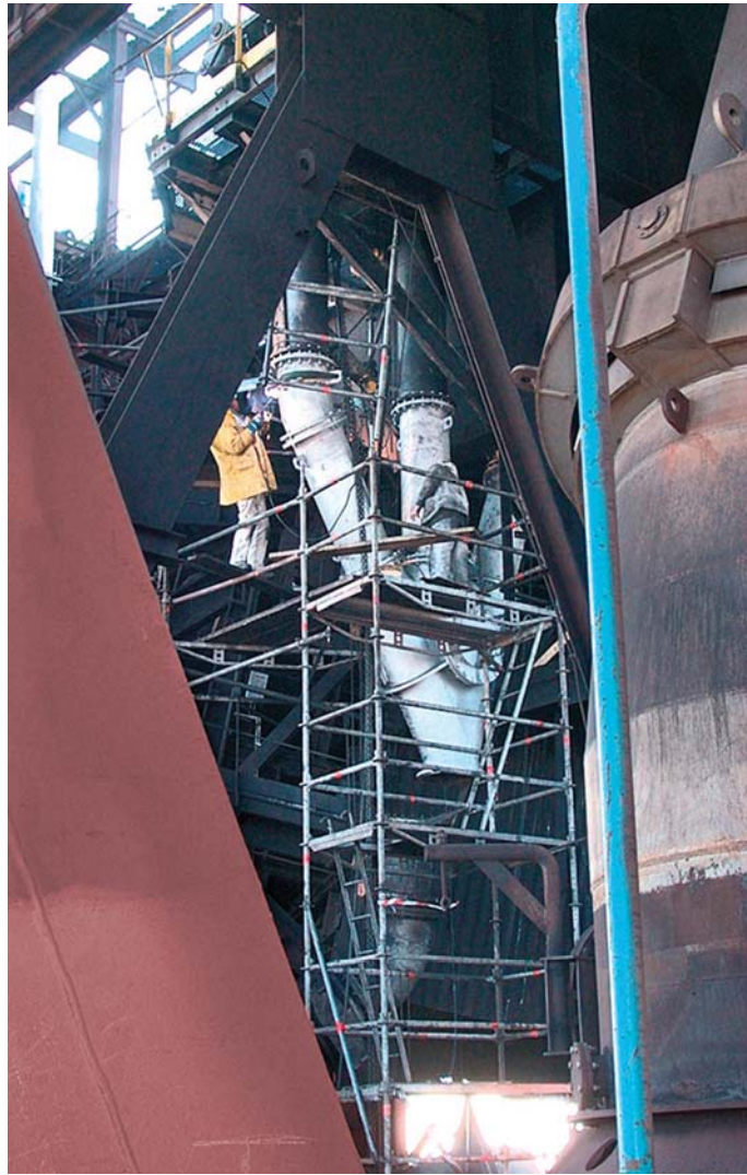
Installation of a pressure compensating pipe at the blast furnace – the self-supporting structure of KALMETALL-W 100 30+6 hard overlay welding has a diameter of 450 mm
