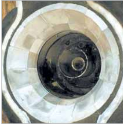
Burner cone made of KALSICA-N in a power plant
