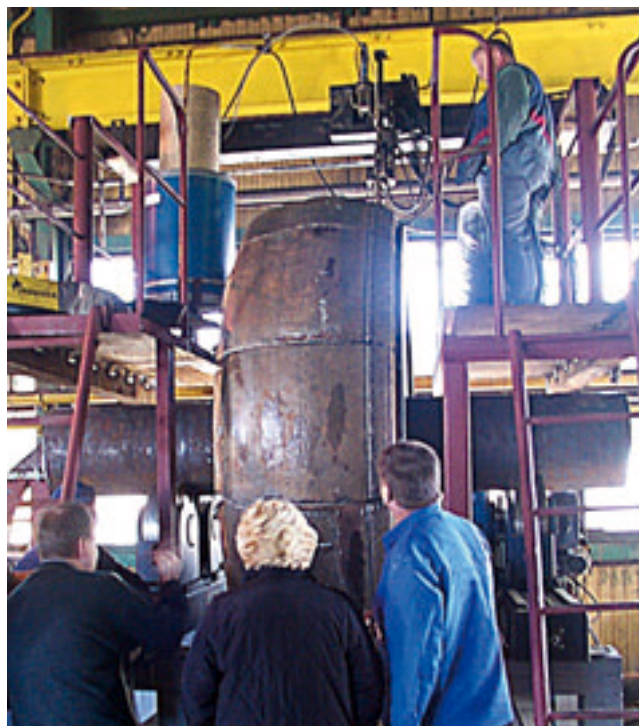
Fig. 18: The Kalenborn service warrants efficient regeneration of grinding rollers with KALMETALL-W 100 hard overlay welding
