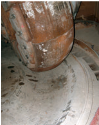
Abb. 10: Grinding elements of roller mills are subject to enormous wear; this is true for both the grinding rollers and the grinding tables
