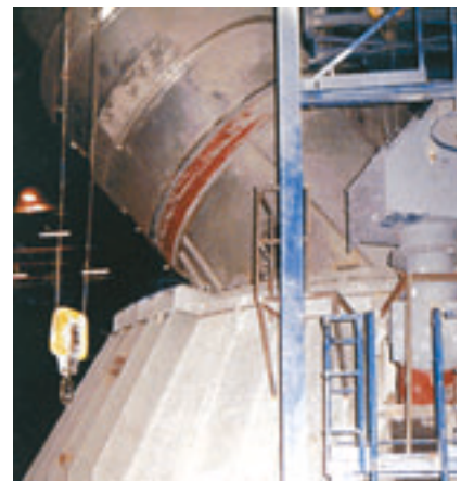
Fig. 9: Protection for a raw meal roller mill: KALCRET installed in the outlet system, KALMETALL-W 100 used as the mill lining
