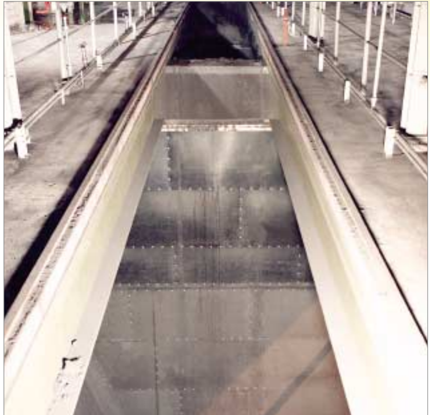
KALEN lining installed in a large German coal-fired power station. The material in the bunker is fine coal.
