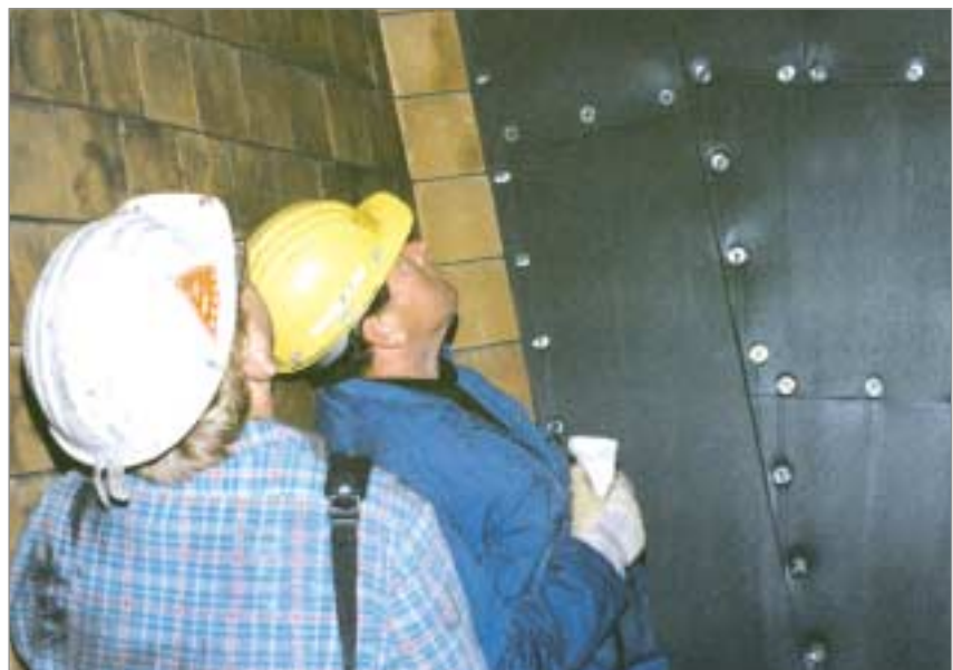
Lining combination in a large fine coal bunker: The surfaces subject to different wear have been protected with due regard to the stress to which they are exposed, here e.g. with KALCERAM and KALEN.
